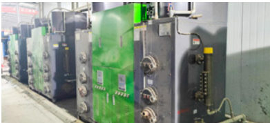
In the Jiangsu Yilu Expressway project by CCCC Second Harbor Engineering, steam was used to replace diesel during boiler combustion, and clean energy biomass fuel was adopted, so that net CO 2 emissions approached zero
