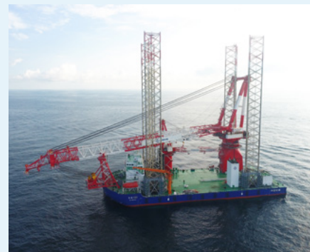
Offshore Wind Power Installation Platform "Haifeng 1001"
